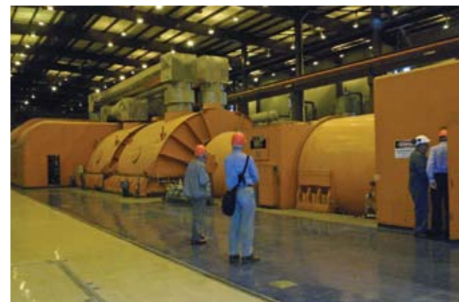
Turbine housing, Newport Power Station
