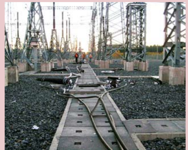
Damaged candlestick-style live tank circuit breakers at power plant, Chile Source: ASCE Technical Council on Lifelines Earthquake Engineering (TLCEE)
