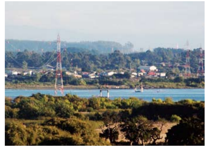
Damaged power transmission towers across the Bio Bio River, Chile Source: Mark Pierepiekarz, MRP Engineering
